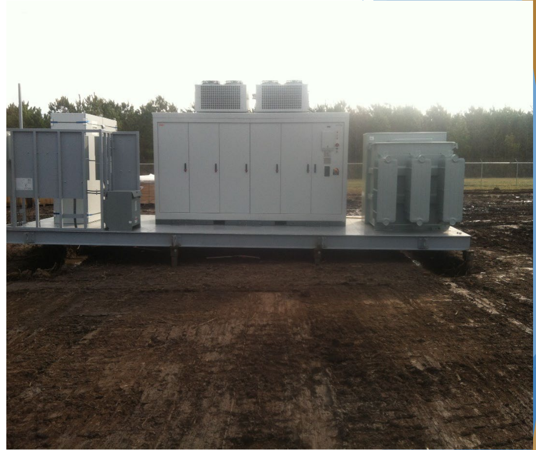
Inverters are installed to convert DC power to AC power.
