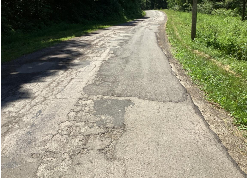
PHOTO 9: Pavement distress (severe pothole, alligator cracking, delamination, edge failure, and patching) on Dixon Run Road, looking west.
