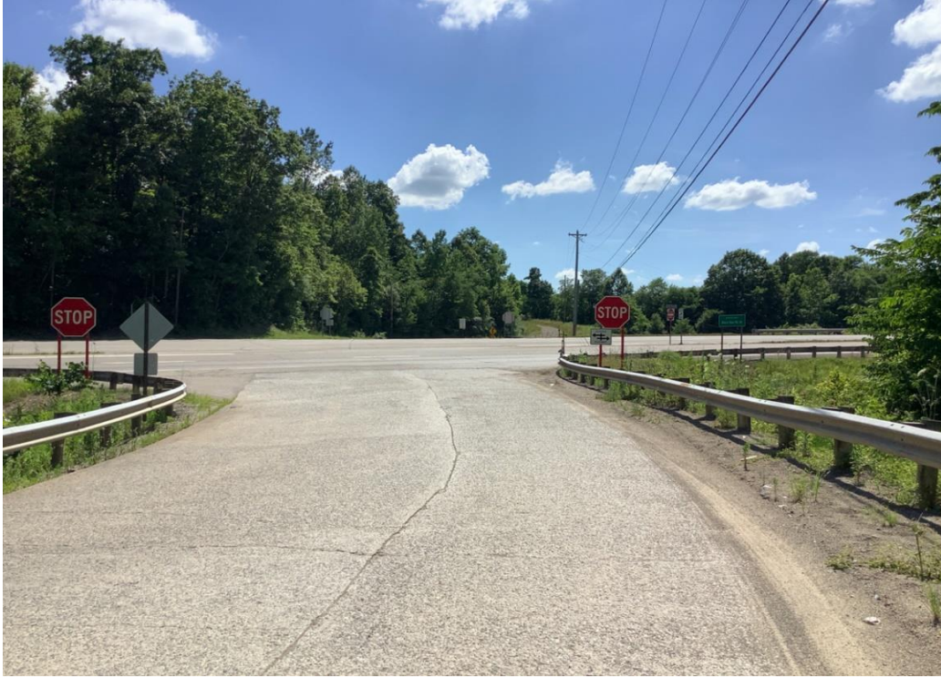
PHOTO 22: Pavement over Bridge 4000668 on Dixon Run Road and intersection with US35, looking west.
