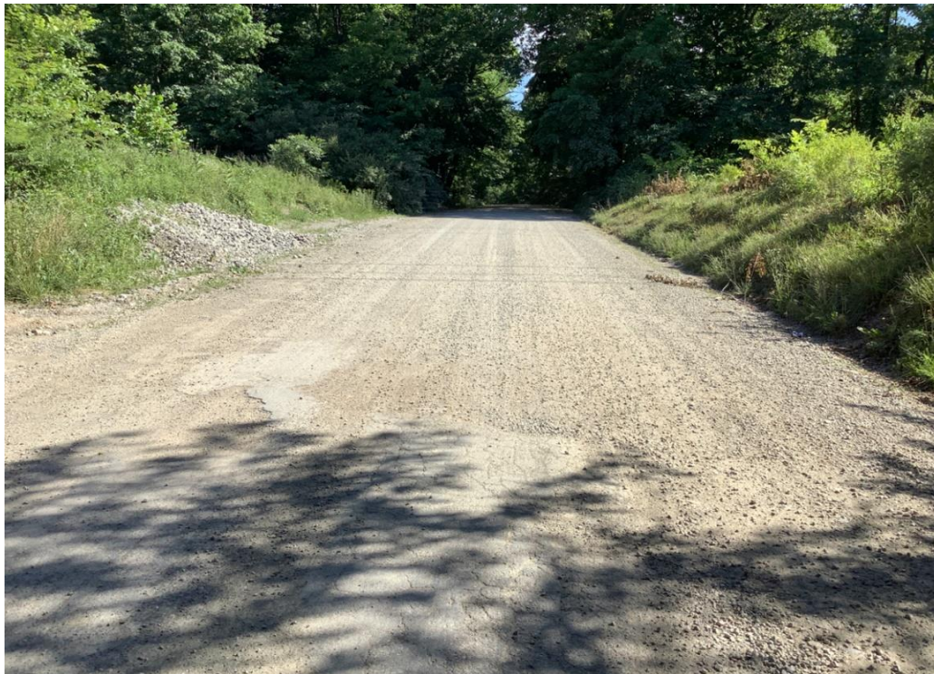
PHOTO 30: Transition from asphalt pavement to aggregate pavement on Luther Jones Road, looking south.
