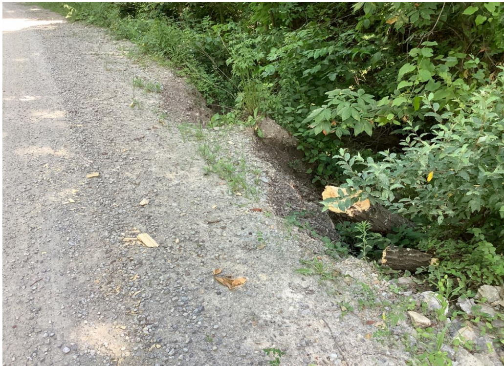
PHOTO 32: Localized embankment erosion on south side of pavement on Luther Jones Road, looking south.
