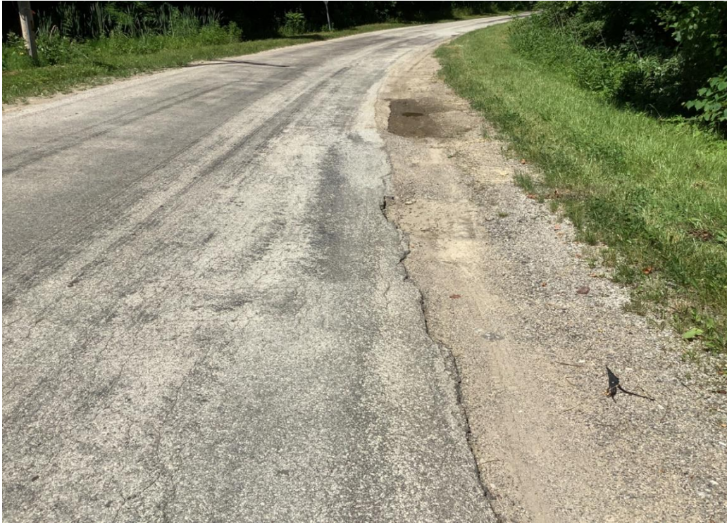
PHOTO 19: Pavement distress (edge and shoulder failure) on Dixon Run Road, looking north.
