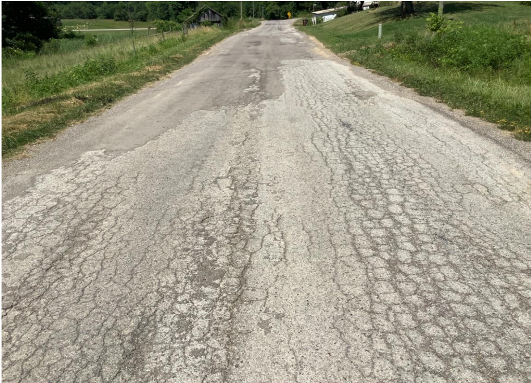
PHOTO 17: Pavement distress (severe alligator cracking and patching) on Dixon Run Road, looking north.
