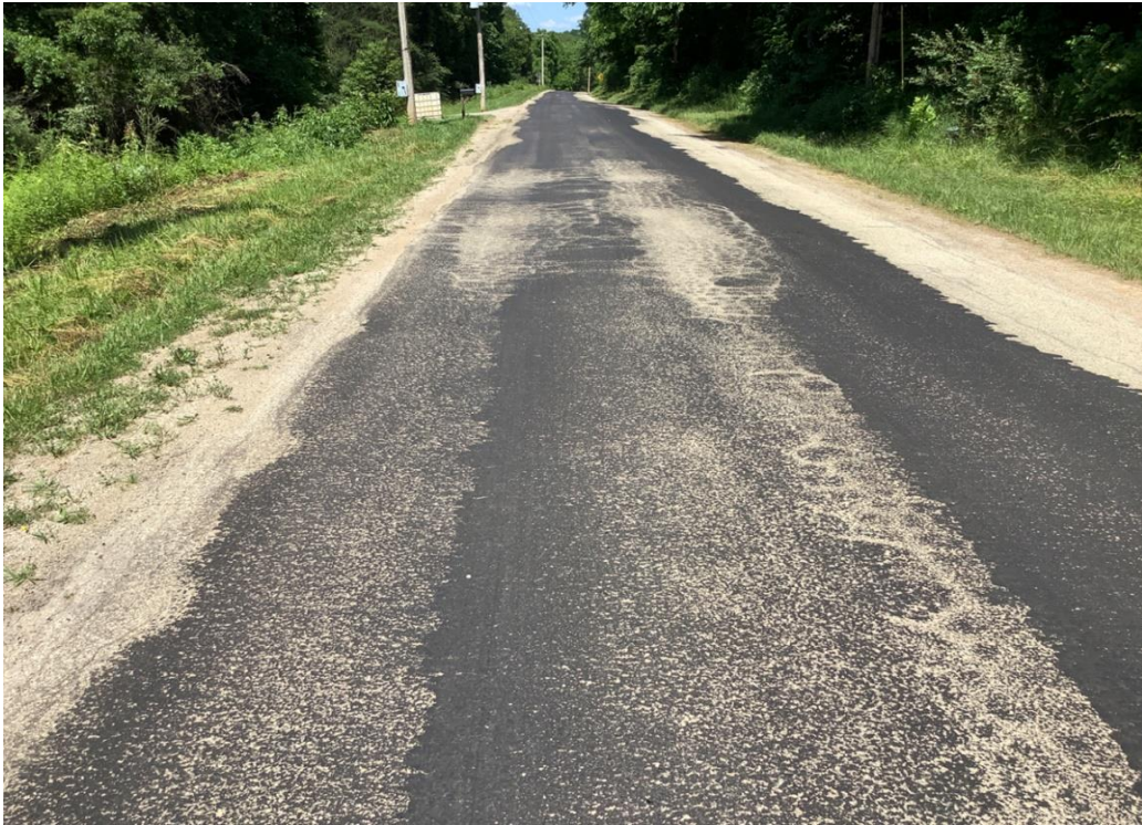
PHOTO 13: Pavement distress (severe rutting and bleeding) on Dixon Run Road, looking north.
