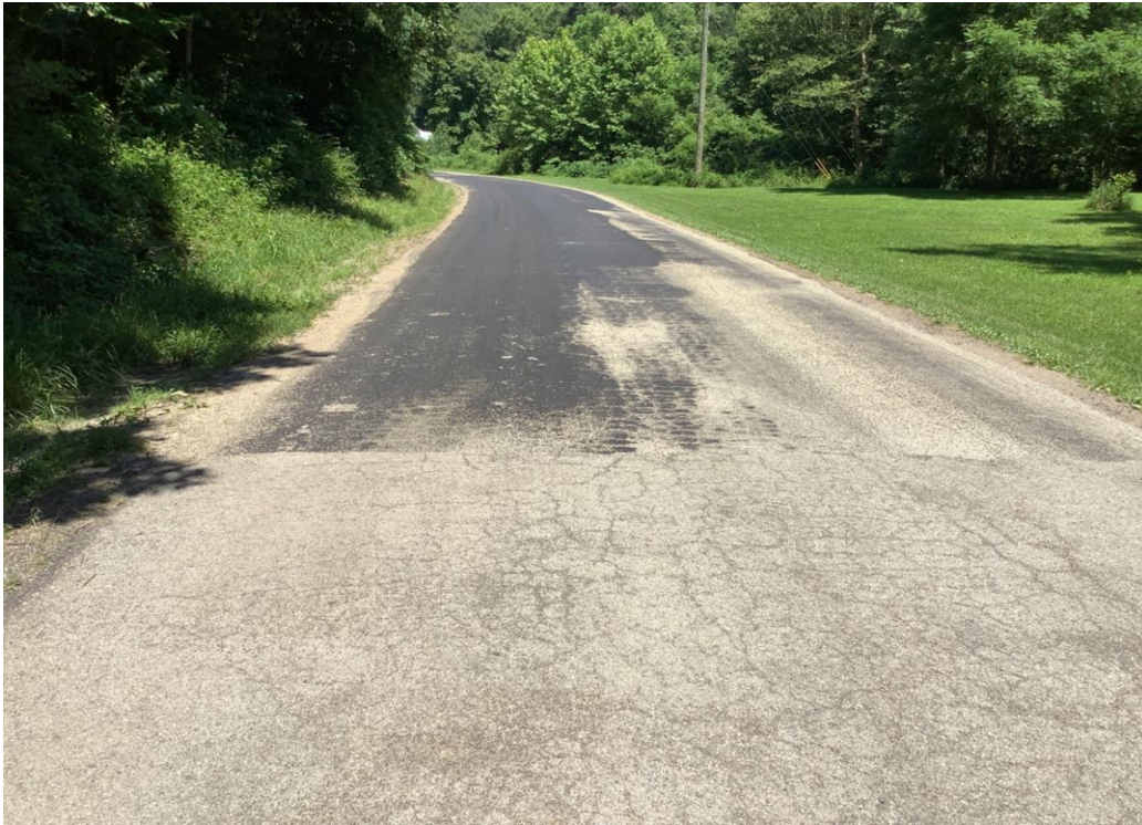
PHOTO 7: Pavement distress (severe bleeding) on Dixon Run Road, looking east.
