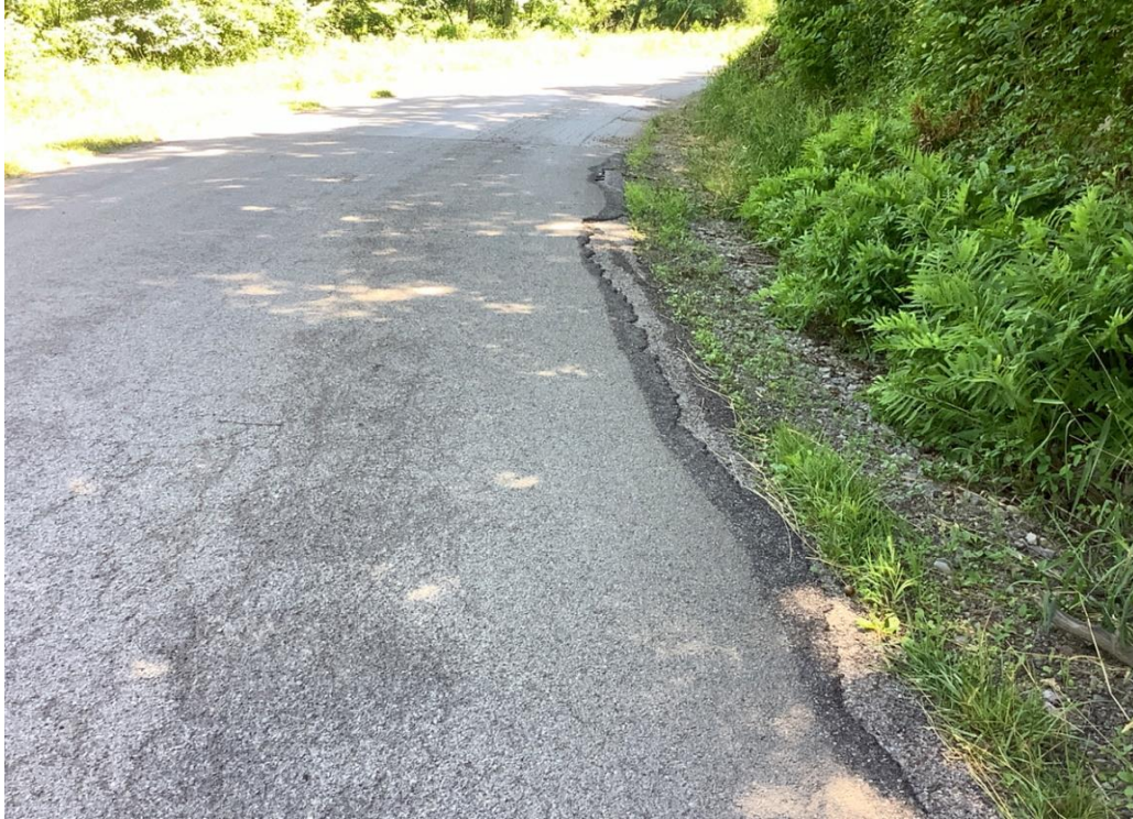
PHOTO 5: Pavement distress (edge deterioration) on Dixon Run Road, looking south.
