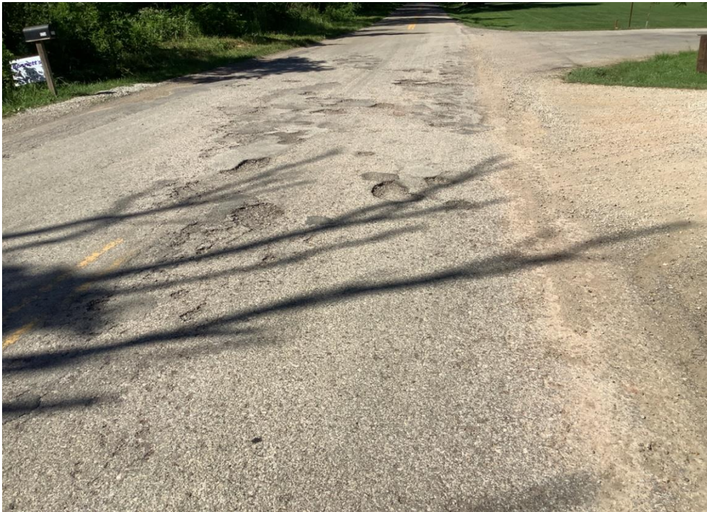
PHOTO 25: Pavement distress (severe delamination, potholes, and patching) on Keystone Furnace Road, looking north.
