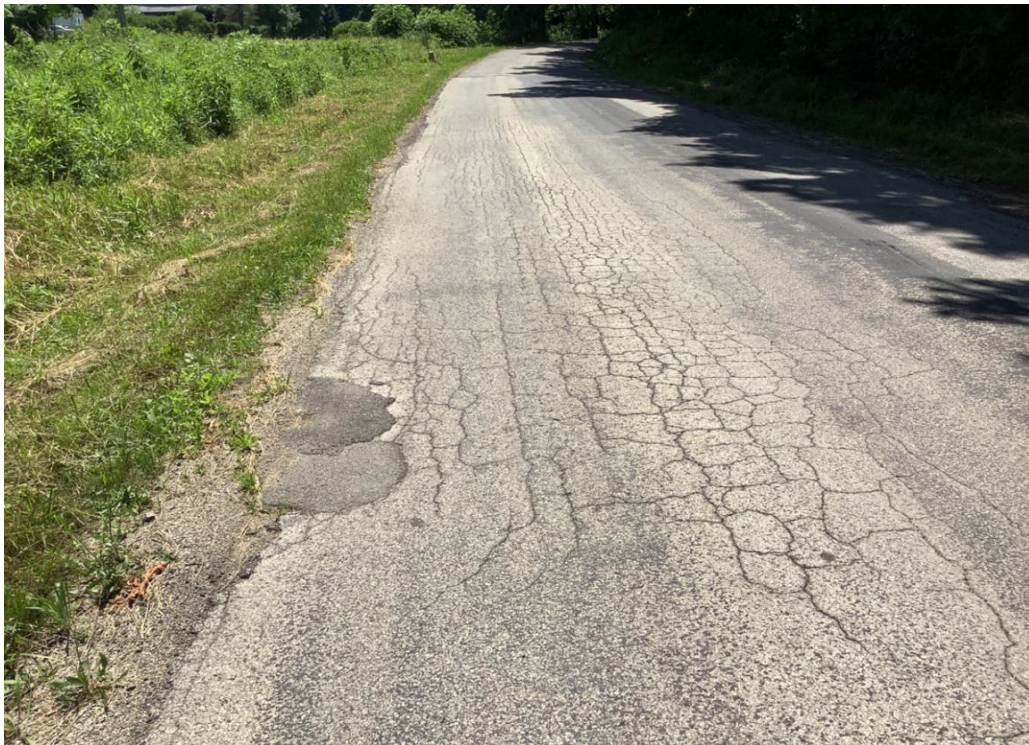
PHOTO 6: Pavement distress (alligator cracking and pothole repair) on Dixon Run Road, looking south.
