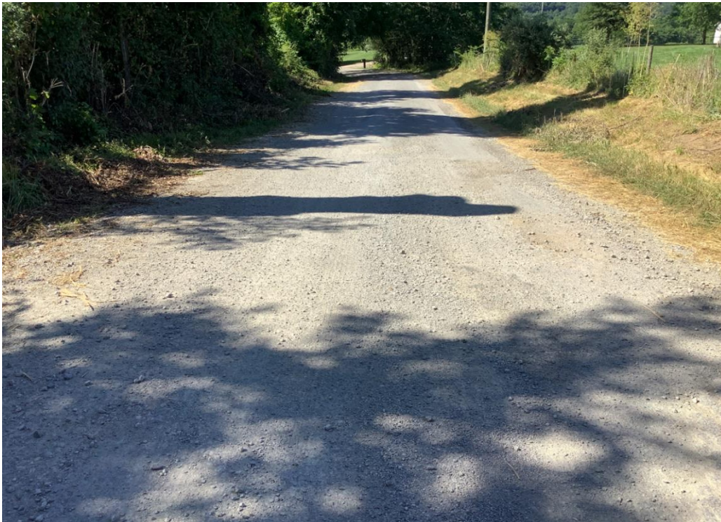
PHOTO 26: Typical pavement distress (potholes, rutting and gravel-filled potholes) for asphalt section of Luther Jones Road, looking north.
