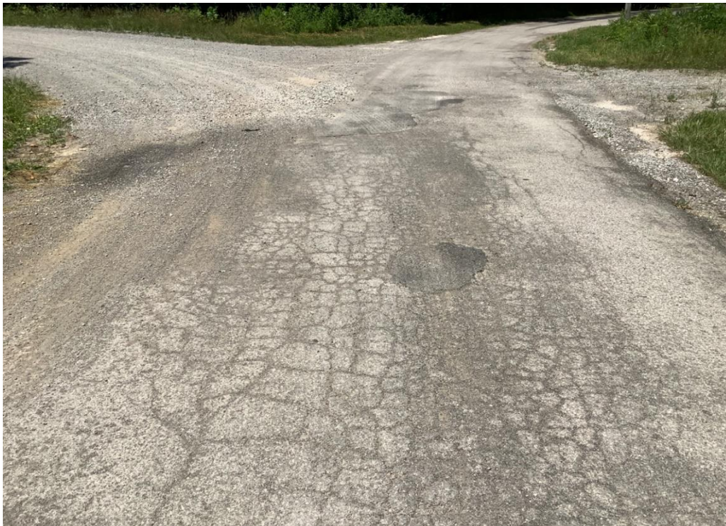
PHOTO 2: Typical pavement distress (alligator cracking and pothole repair) on Dixon Run Road, looking north.
