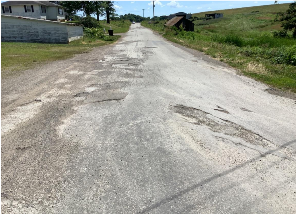
PHOTO 15: Pavement distress (severe pothole, alligator cracking, rutting, and patching) on Dixon Run Road, looking south.
