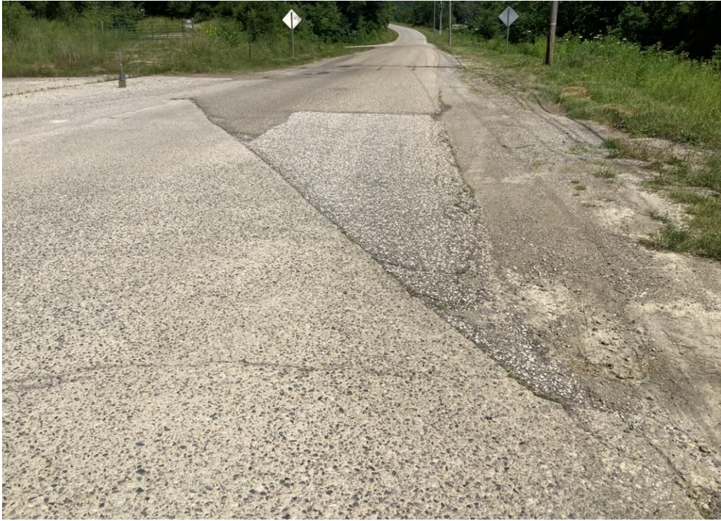
PHOTO 21: Transition from concrete pavement to asphalt pavement on Dixon Run Road, looking east.
