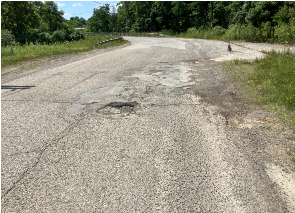
PHOTO 20: Pavement distress (severe pothole, alligator cracking, delamination, edge failure, and patching) on Dixon Run Road, looking west.
