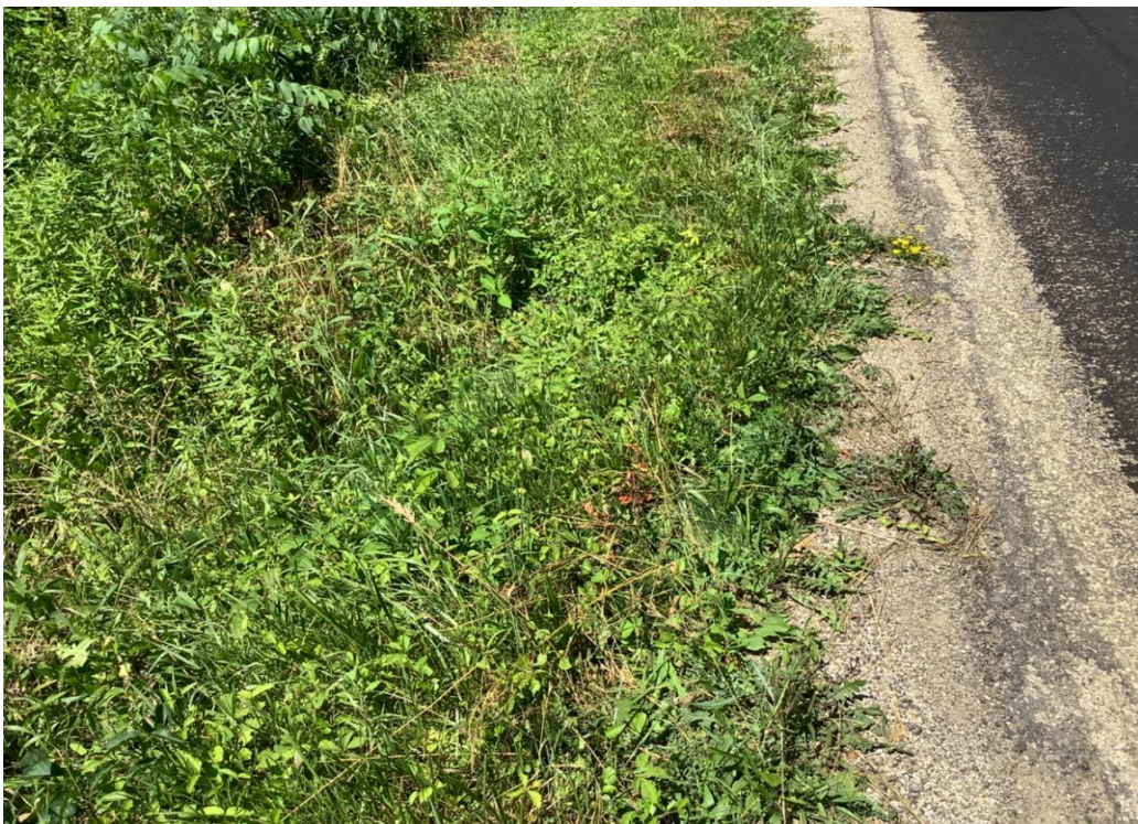
PHOTO 14: Embankment erosion on west side of pavement on Dixon Run Road, looking north.
