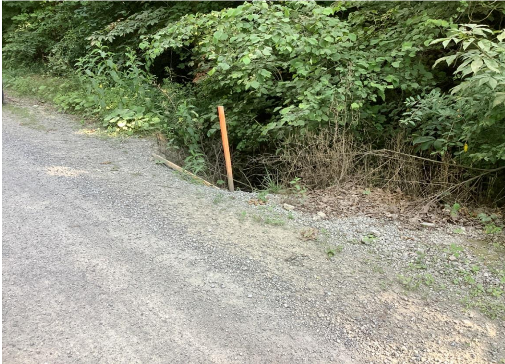
PHOTO 35: Localized embankment erosion on south side of pavement on Luther Jones Road, looking south.
