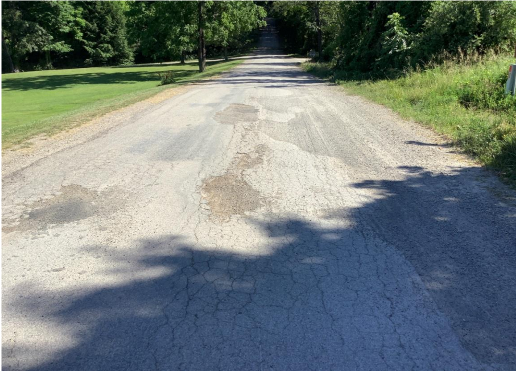
PHOTO 27: Typical pavement distress (severe rutting, alligator cracking, and gravel-filled potholes) for asphalt section of Luther Jones Road, looking south.
