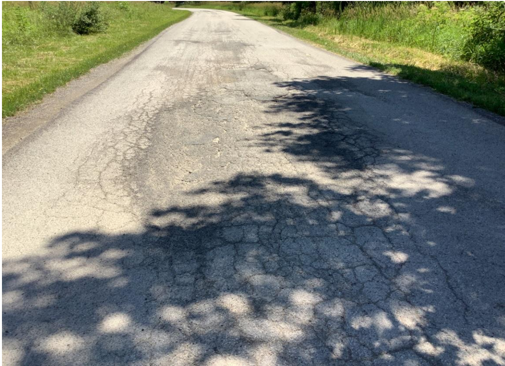
PHOTO 3: Pavement distress (severe pothole, cracking and base deterioration) on Dixon Run Road, looking south.
