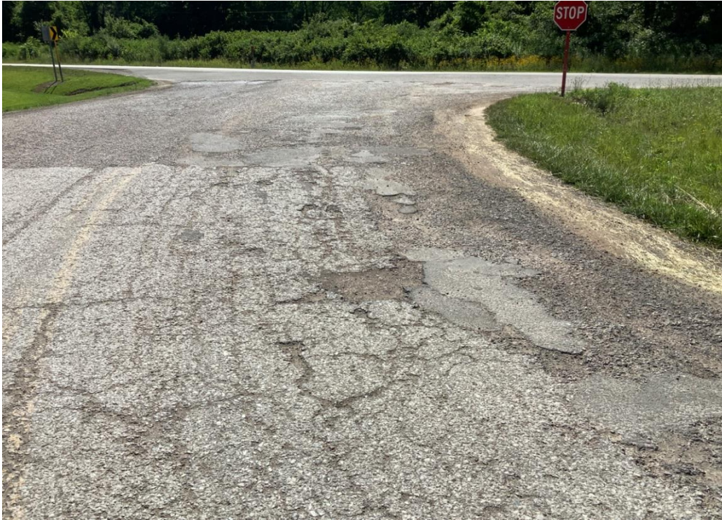
PHOTO 23: Pavement distress (severe delamination, raveling, and patching) on Keystone Furnace Road, looking west.
