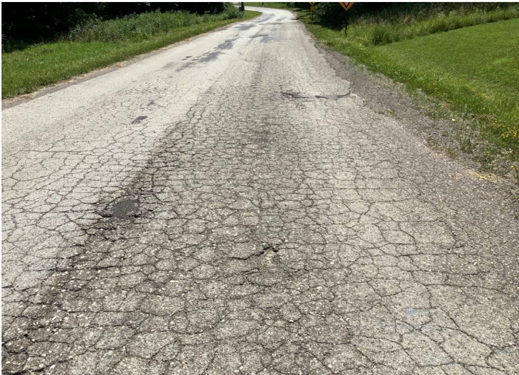
PHOTO 18: Pavement distress (severe alligator cracking and edge failure) on Dixon Run Road, looking south.
