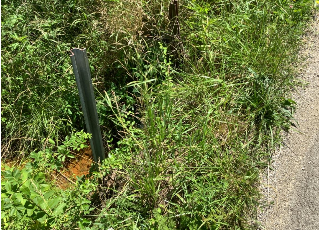
PHOTO 11: Embankment erosion on south end of culvert on Dixon Run Road, looking west.
