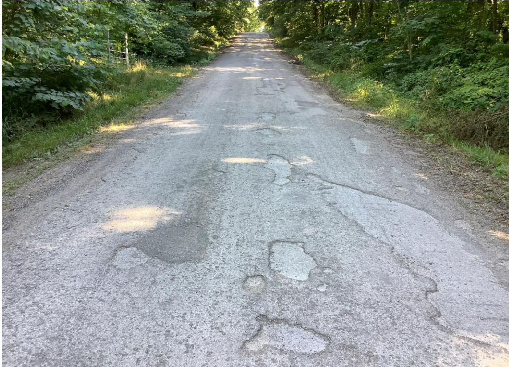
PHOTO 29: Typical pavement distress (severe delamination and edge failure) for asphalt section of Luther Jones Road, looking south.
