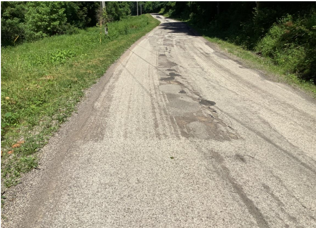
PHOTO 12: Pavement distress (severe delamination, potholes and patching) on Dixon Run Road, looking east.
