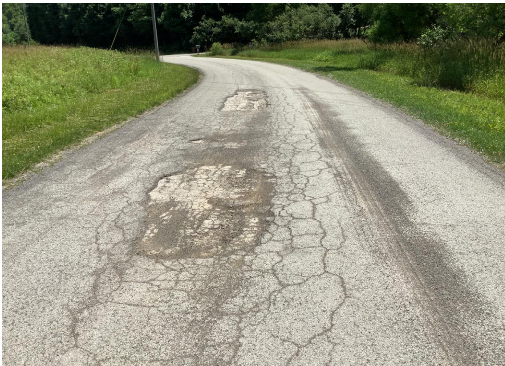
PHOTO 4: Pavement distress (severe pothole and delamination) on Dixon Run Road, looking south.
