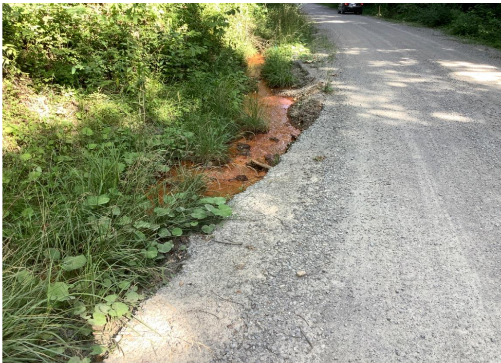
PHOTO 34: Flow from spring causing embankment erosion on north side of Luther Jones Road, looking east.
